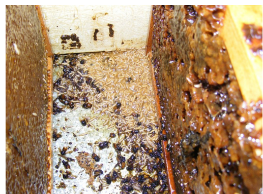
Damage done by SHB
